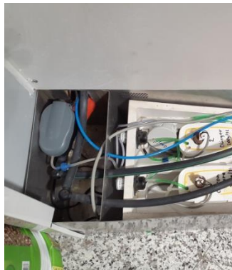
Medium sized pumping station with solenoids, filter and two fertigation tanks and air compressor integrated in a gutter below the green wall
