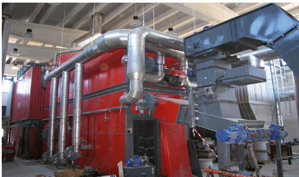
Picture 5. Mobile grid boiler for producing electricity from woody biomass Source: (Fiusis website)
