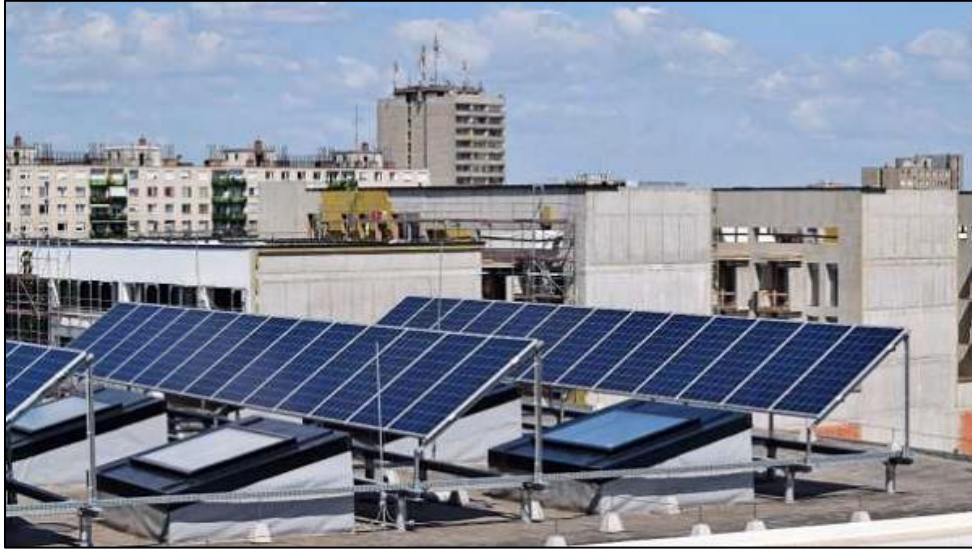
Figure 1: Photovoltaics system at roof 1
